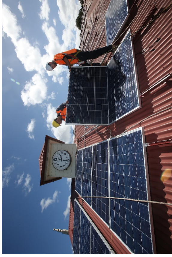
Image: Solar panels are installed on the roof of the pavilion at Sydney Park
